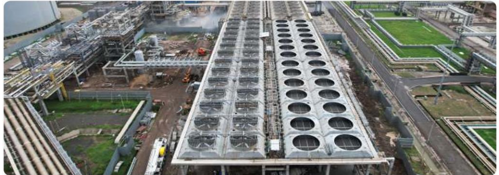
Exhibit 1: Regas capacity expansion at Dahej terminal
