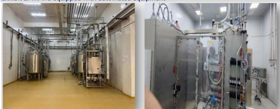
Exhibit 2. ...And equipped with automated equipment
